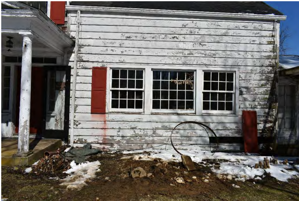
Figure 73. Photograph of 248 Stickles Pond Road, Building #5, detail of east addition facing north.
