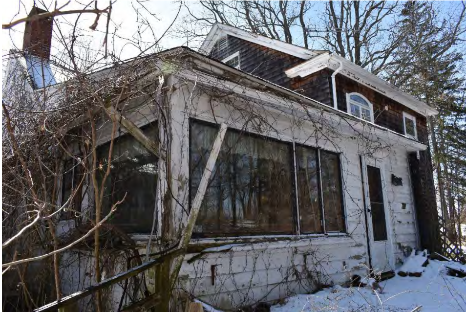
Figure 72. Photograph of 248 Stickles Pond Road, Building #5, facing southwest showing detail of rear of central addition.
