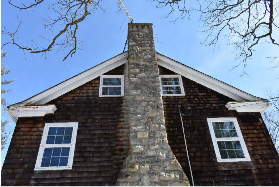
Figure 70. Photograph of 248 Stickles Pond Road, Building #5 facing northeast showing detailed view of stone chimney.
